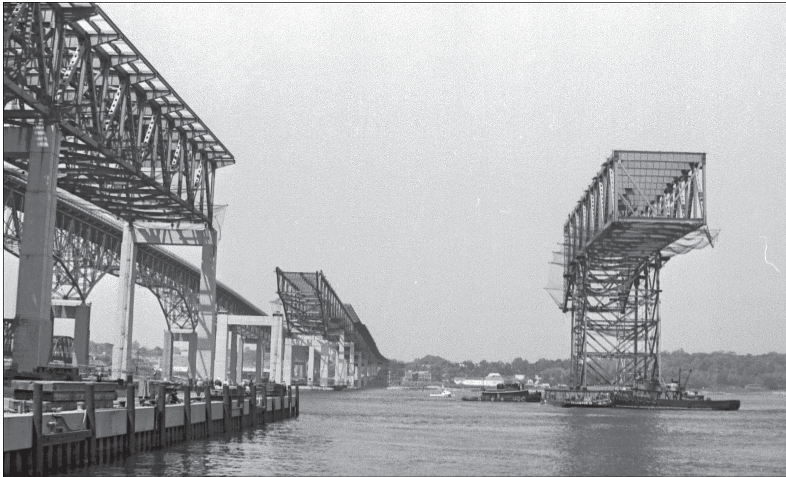
An 1,100-ton truss span for the second Gold Star Memorial Bridge is floated into place on June 2, 1972, after it was built nearby at Whaling City Dredge and Dock in Groton. DAY FILE PHOTO
